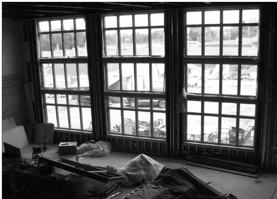
View of the Multi-Purpose Room from the second floor, showing the room's 2-story-high windows, which will look out on the existing SAD 22 multi-purpose field.
