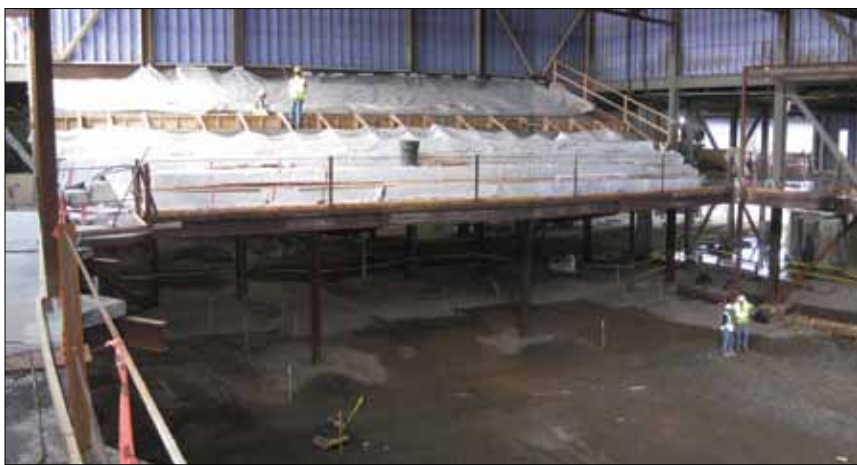
Cement has been poured for the bleachers in the new performing arts center.
